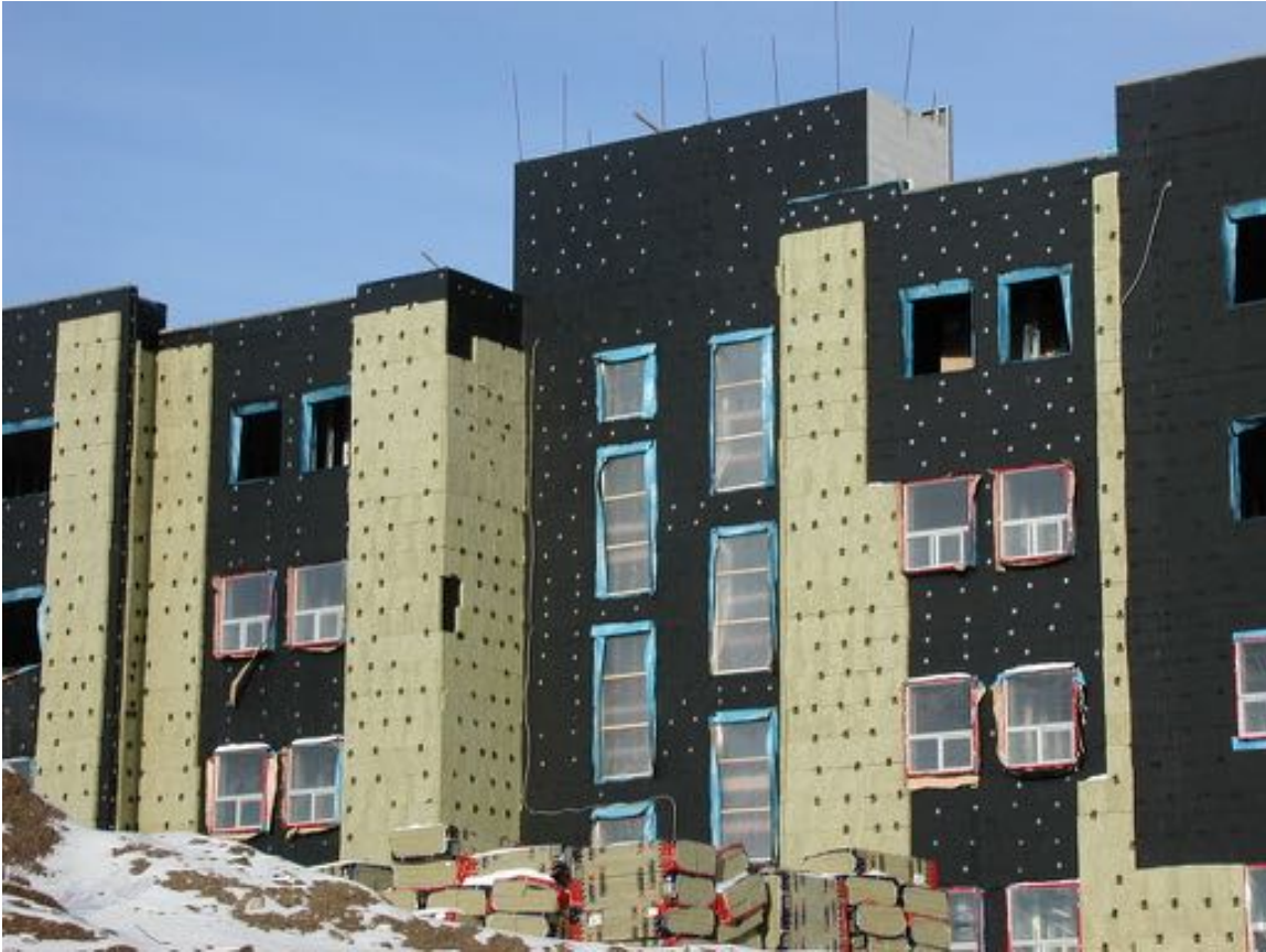
Rockwool semi-rigid board insulation used as continuous exterior insulation in an institutional building over a fluid-applied asphaltic air-water barrier over CMU
